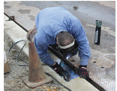
Modifications can be necessary, but must be carefully evaluated as to not harm the scale's structural integrity
