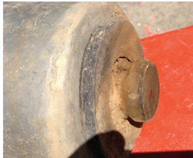
Insufficient maintenance in the past accelerates physical wear to the load cells and shortens their life
